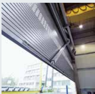
Wind Protection System (WPS)
